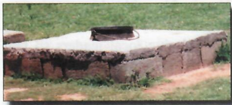
One of the wastewater pits built by Youth21 for the community of St. Michael's (Pic by L. Lejakane).
